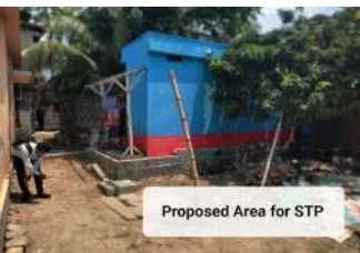
Project Name: Bastuhara Colony Capacity: 30 m 3 /day Location: Bastuhara, Khulna
