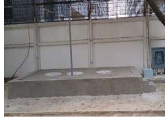
Project Name: Bashundhara Group Chairman's Residence Capacity: 10 m 3 /day Location: Bashundhara R/A
