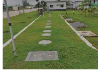
Project Name: 62 Bengal Capacity: 100 m 3 /day
